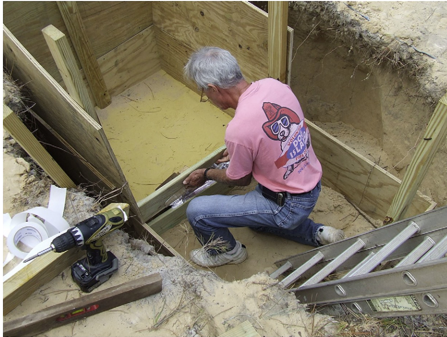
Fig. 2. Construction of the layered sand column within the plywood box. Beginning at 2 m depth, different colors of sand were layered and packed. The open side of the box was closed with boards as the level of sand rose. The yellow sand layer is shown in place here. Once complete, all sides around the box, and the work pit were refilled with sand. (For interpretation of the references to color in this figure legend, the reader is referred to the web version of this article.)
